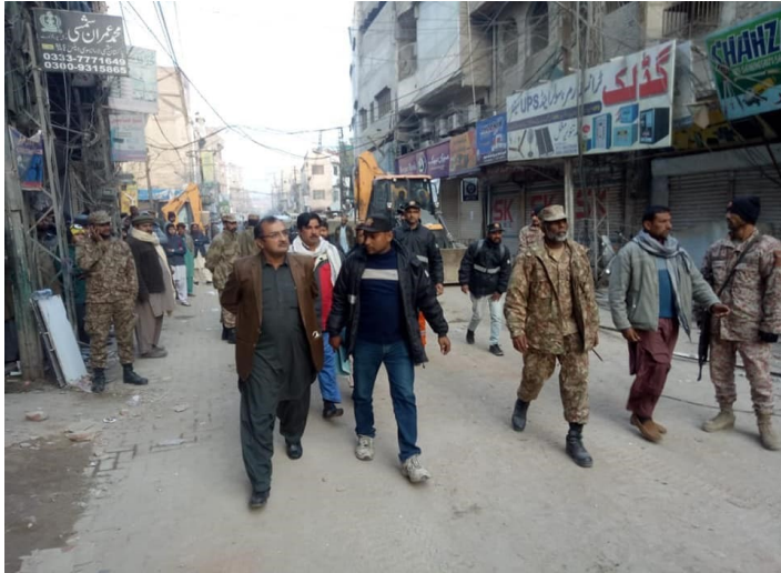
Sukkur: Rescue Ops at collapsed building in Sukkur
