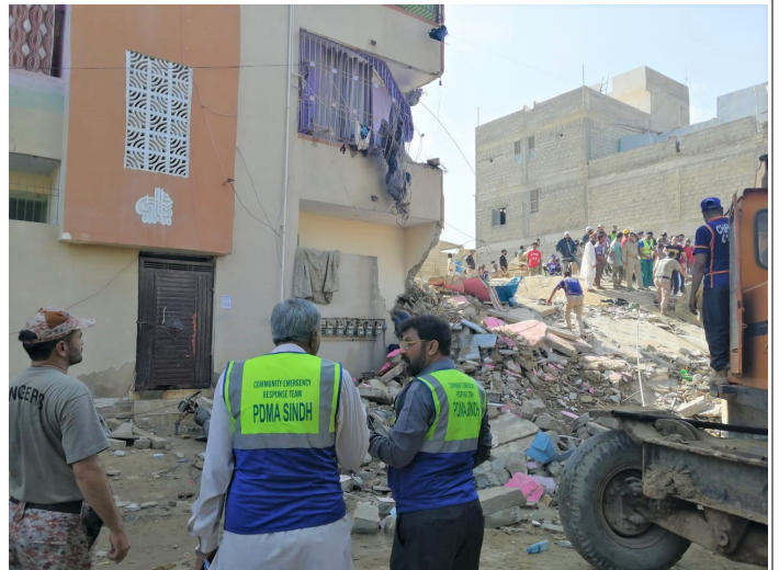
Karachi: PDMA Sindh Rescue ops at collapsed building in Korangi
